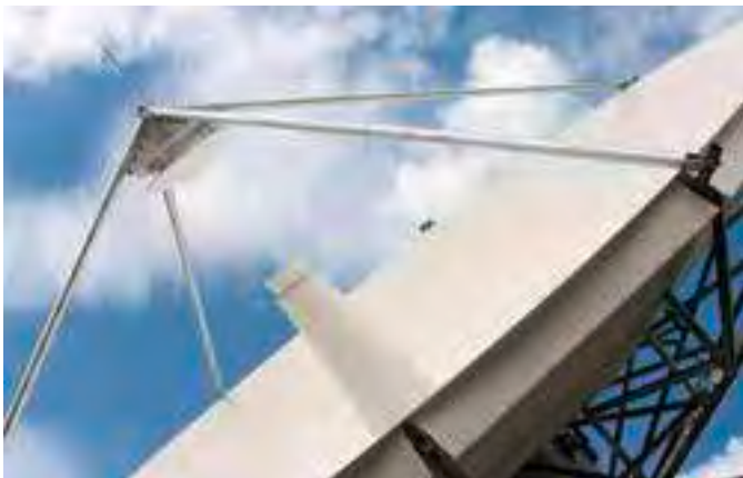
9.5 m C-band antenna installed at Munich site.
